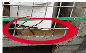
Broken round steel mesh
