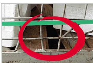
Board lost or broken
