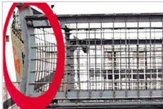
Deformed push-fit bracket/corner column
